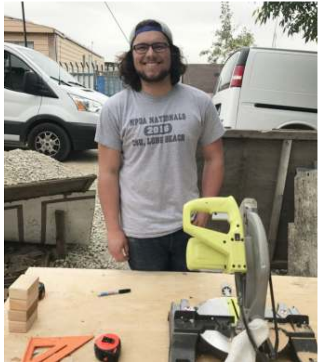
A Concordia University student ready to start to work cutting lumber. They built a home for two young boys and their mom in El Maclovio Rojas, Baja California.
