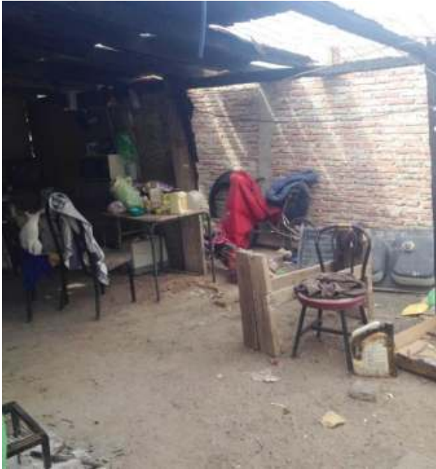
Pictured above is a home in the Sonora Desert that is in need of many repairs, including the roof. A new home is scheduled to be built for the family in the near future.
