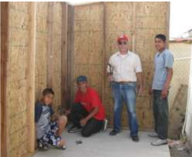
With Pastor Romelio is Rafael and two youth from Principe de Paz . They were building new toilet facilities, actually an outhouse with a nice building, they have no sewer available yet.
