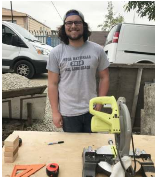
A Concordia University student ready to start to work cutting lumber. They built a home for two young boys and their mom in El Maclovio Rojas, Baja California.
